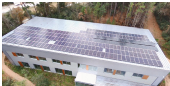
Figure 9. Rooftop solar panels as seen from the north side of the HARC office building. Photo: HARC
